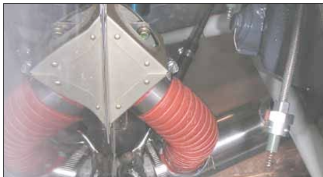
Cabin air ducting using a readily available box from one of the hardware suppliers.
