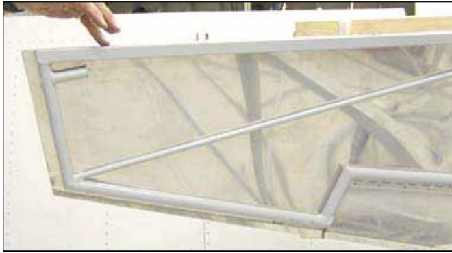
Once the skin is attached to the outside, the interior panels can be screwed directly to the door frame
