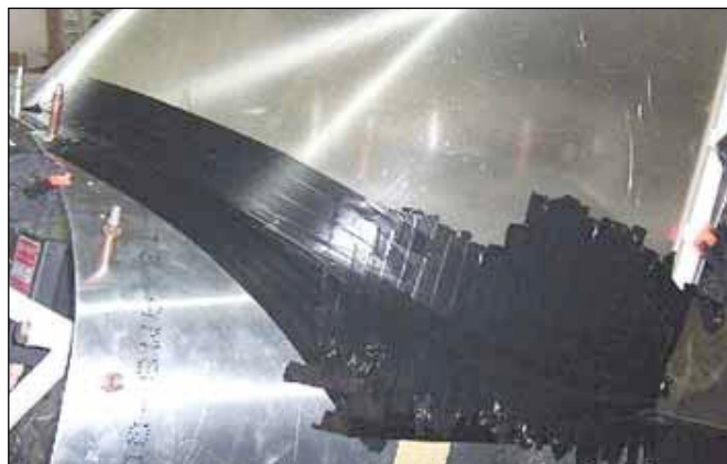
Be sure to put down a "release" surface before applying the fiberglass. This builder used electrician's tape but packing tape or even Scotch tape works fine. Don't even think about not using a release or you'll have everything stuck together.
