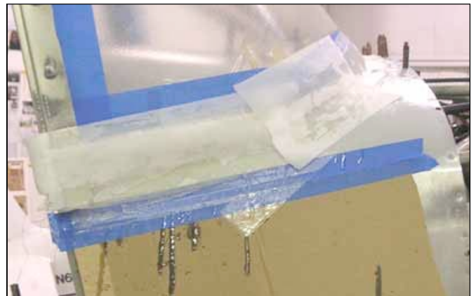
Laying the soaked cloth strips in position is messy and needs two sets of hands. Cover everything in sight to protect it. The material will stretch and conform but be sure to roll out any bubbles and excess resin.
