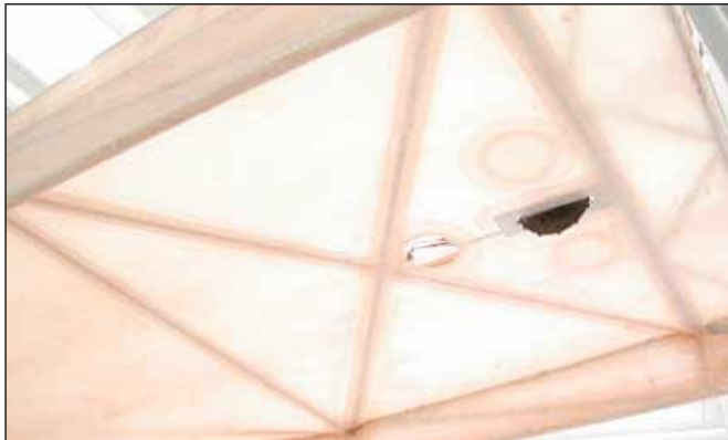
The headliner: a fabric interior requires rings to be glued to it in appropriate places to affix inspection panels.
