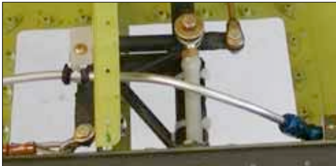
Aileron bellcrank. Here you can clearly see the cable at the bottom of the picture that is connected to the other wing. At the lower right you can see the fuel pump and the transfer line.
