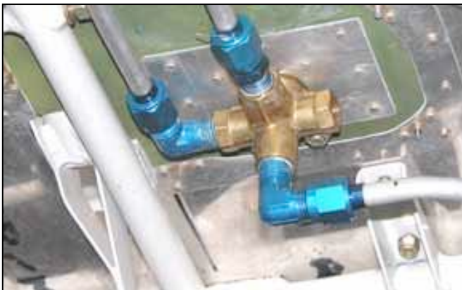
fuel valve plumbing depends entirely on what type of valve you are using and the positions on that valve. A Left-Right-Off-Both is optimum, but many builders opt for a Left-Right-Off only.
